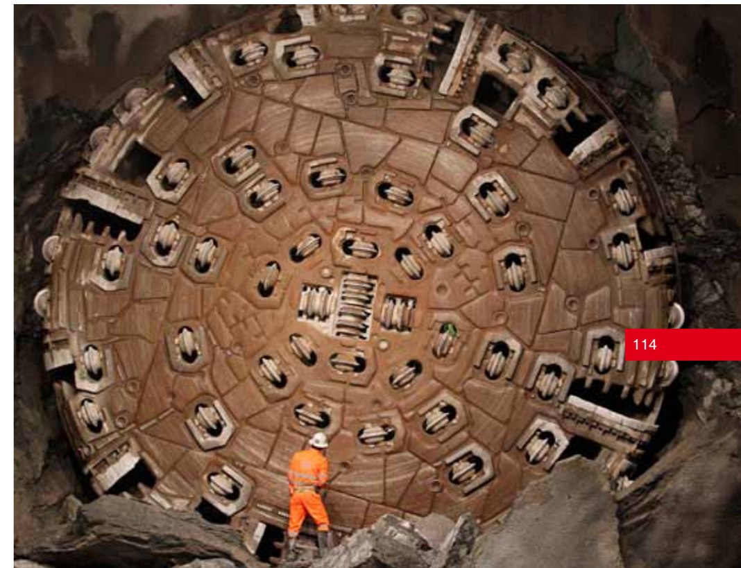
Construction of the Gotthard Base Tunnel: situated beneath the Swiss Alps and expected to open to the public in 2016, the Gotthard Base Tunnel will be the world's longest railway tunnel (57 km). © AlpTransit Gotthard AG
